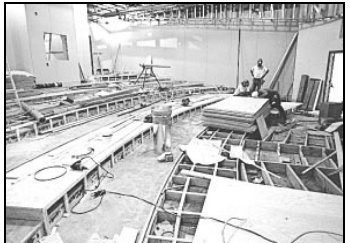
Carpenters give DeTamble Auditorium a facelift in preparation for its conversion to a multimedia and information highway classroom.
